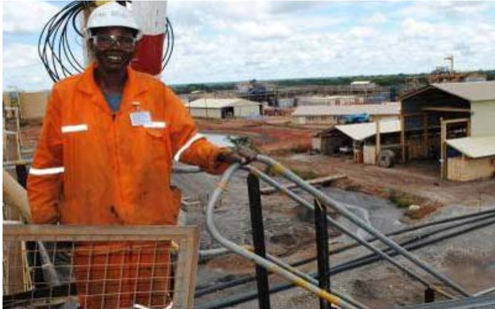
Fitter Jean Tshisola Tshijika at work at Kinsevere's Stage I HMS plant. In the background is the Stage II development
