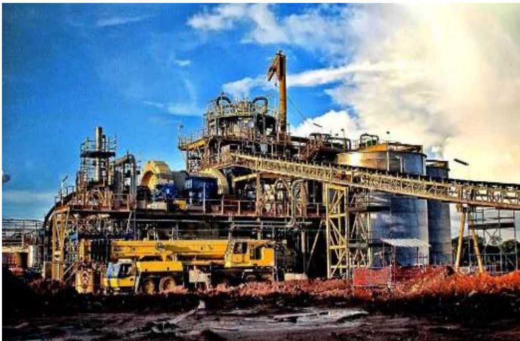
Jan van Schaik's dramatic photo of Stage II under construction shortly after rain had cleared the air
