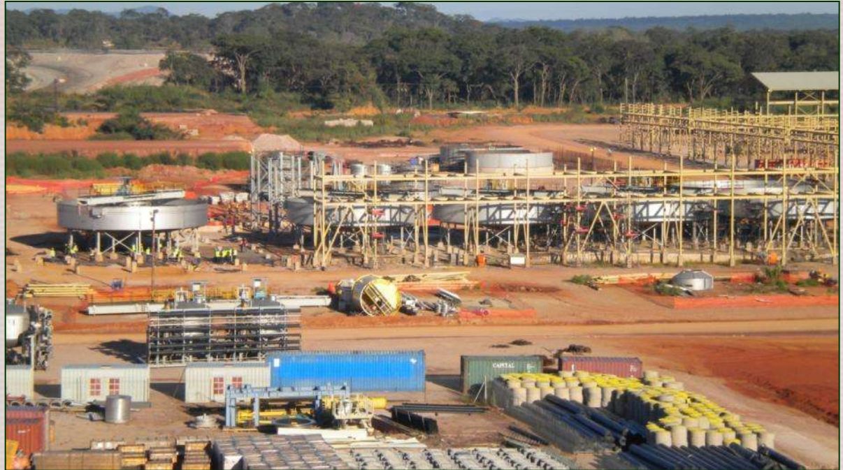
Pipe racks, CCD thickeners & acid tanks
