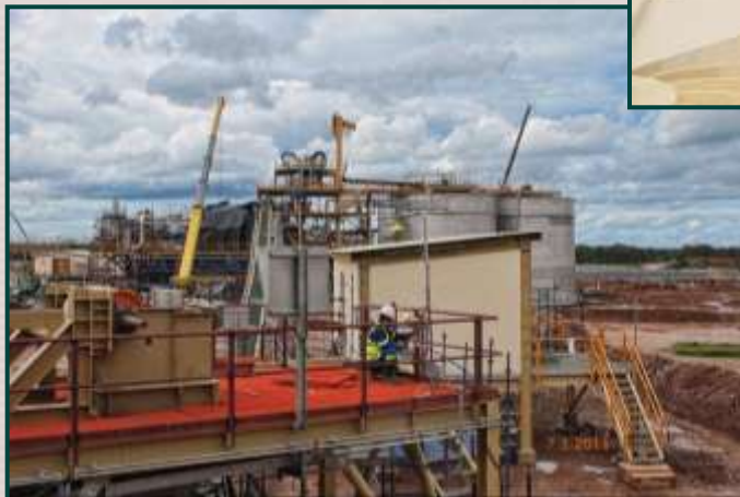
Crusher Mill & Leach Tanks in Background
