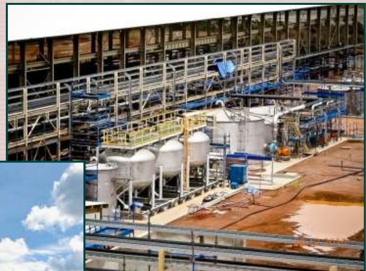
Electro-Winning Building Multi-Media Filters
