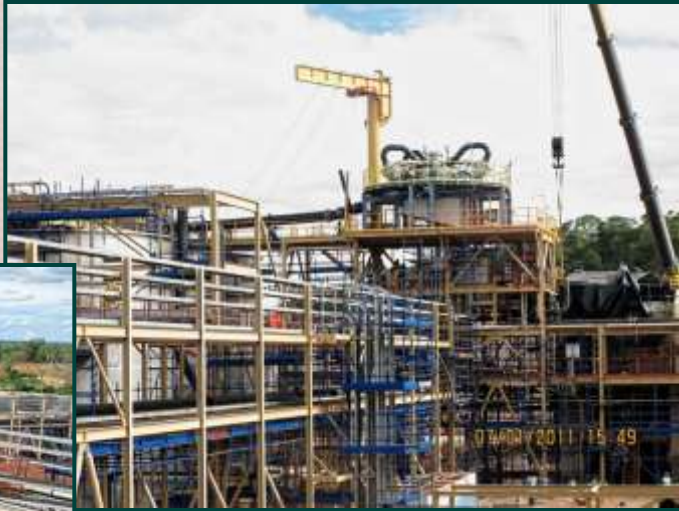
Cyclones & Cyclone Jib Crane
