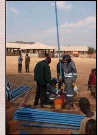
Piping for fresh water well
