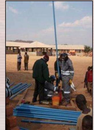
Piping for fresh water well
