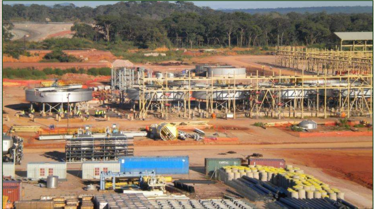
Pipe racks, CCD thickeners & acid tanks
