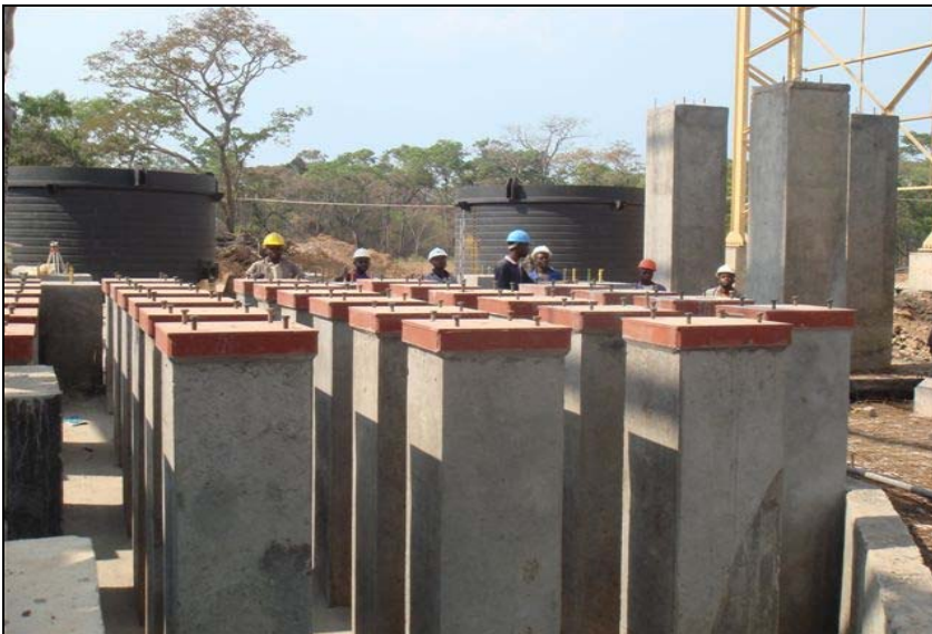
Kinsevere Stage I Electric Arc Furnace Bases with Furnace Shells in Background
