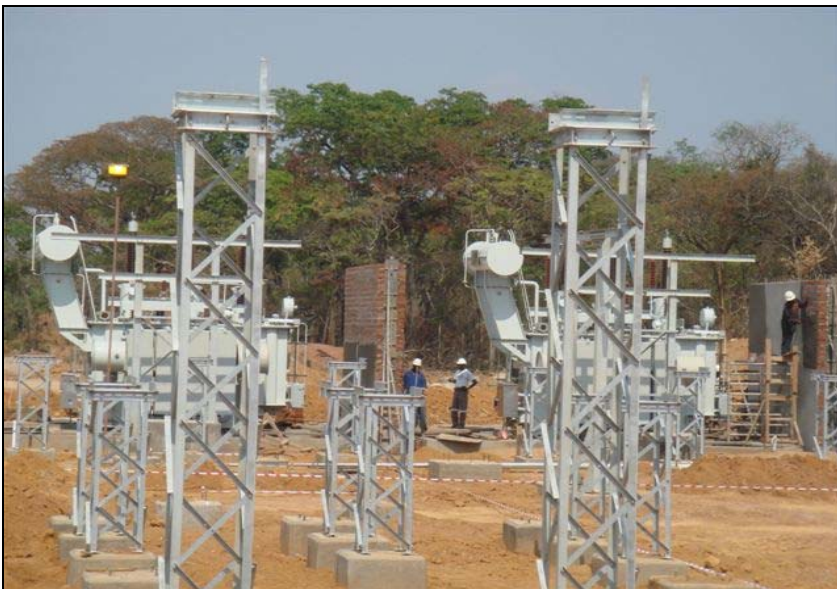
Kinsevere Mine 2 x 30MW 120kV/33kV Step Down Transformers and Switchyard
