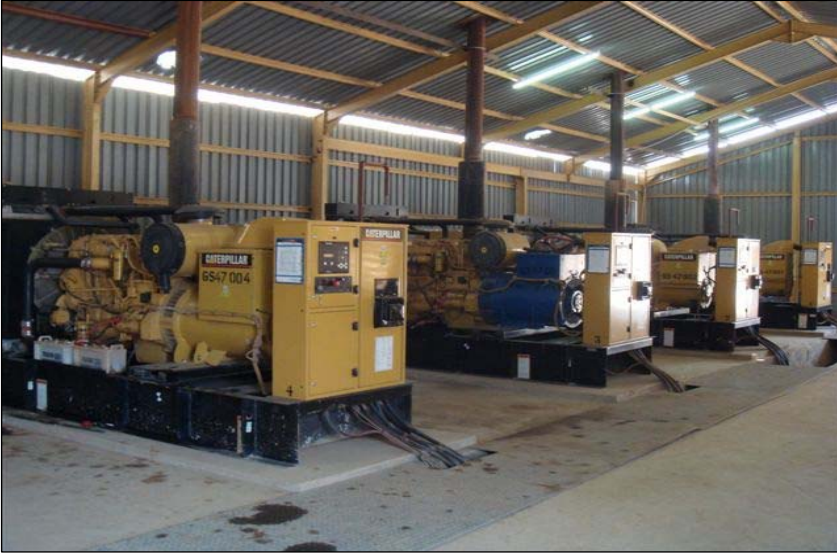
Kinsevere Mine Stage I Power Station – 2MW (temporary diesel generators)
