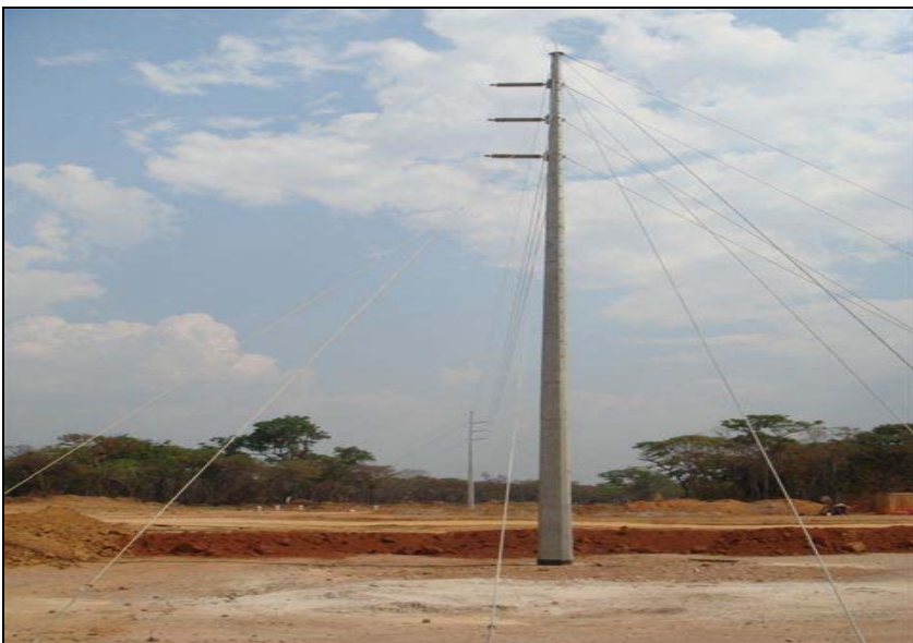
End of 27 km 120kV Transmission Powerline Connecting Kinsevere Mine to DRC Hydro-Electric Grid
